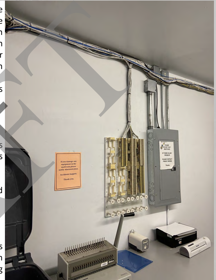
Figure 8-3. Exposed wiring in City Hall
