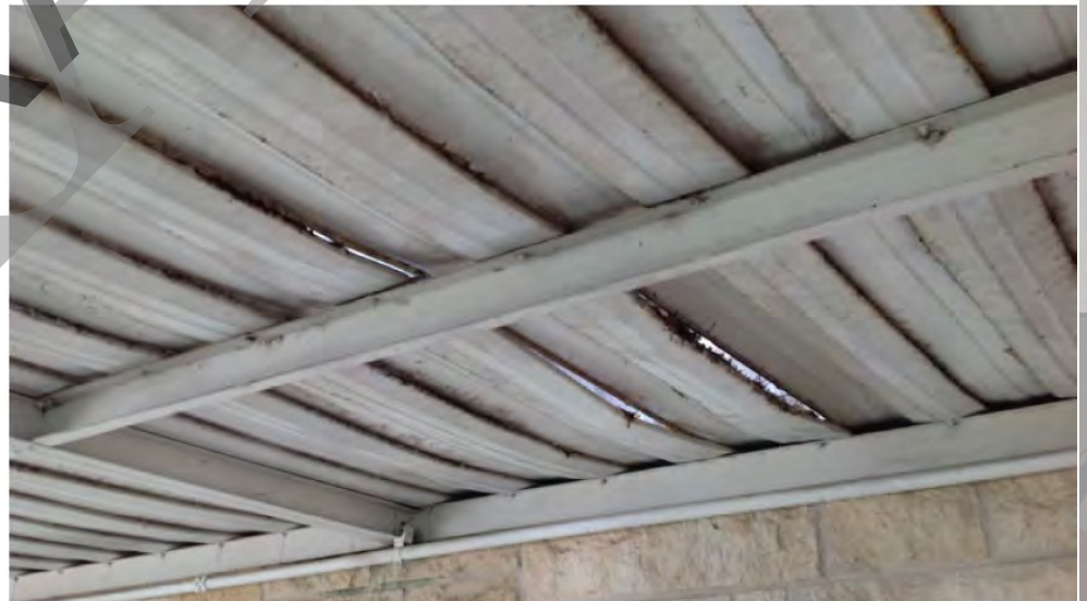
Figure 8-1. The Canopy around the Golf Course Club House. You can see the deterioration and damage that has happened due to weathering.
